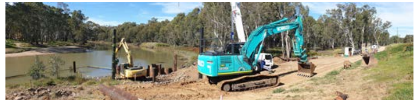
The new $1.1 million boat ramp and floating pontoon is being built on the southern side of the Murrumbidgee River, opposite the Darlington Point Caravan Park and adjacent to the Darlington Point flood levee bank. The project is funded through a $450,000 grant through the NSW Government's Boating Now Program, with the remainder funded by the NSW Government's Stronger Communities Fund.
