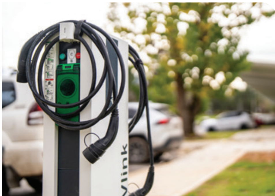
Electric vehicle charging station, Brolga Place, Coleambally.
