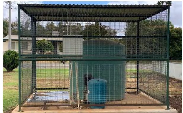
Figure 11 – Water tank enclosure
