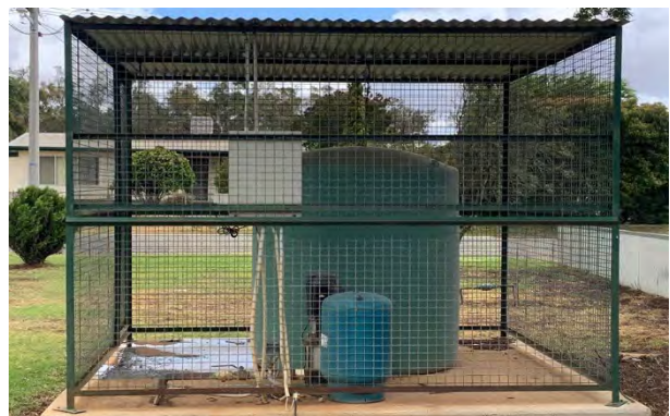
Figure 11 – Water tank enclosure
