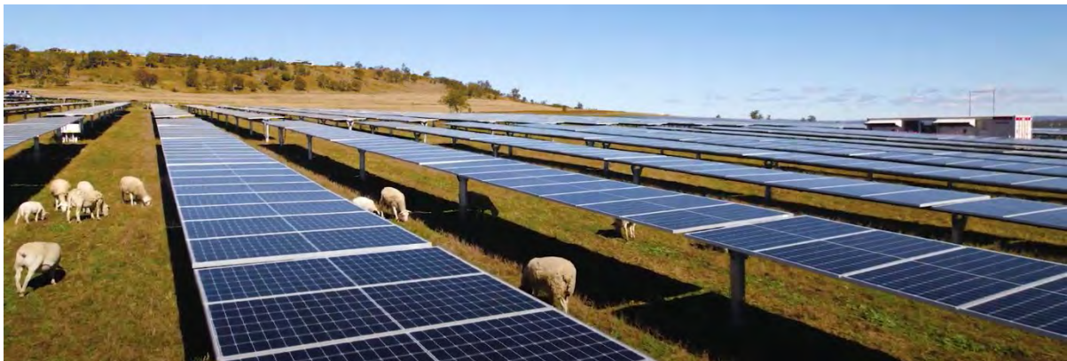
Nextracker SAT system – panels flat at midday
